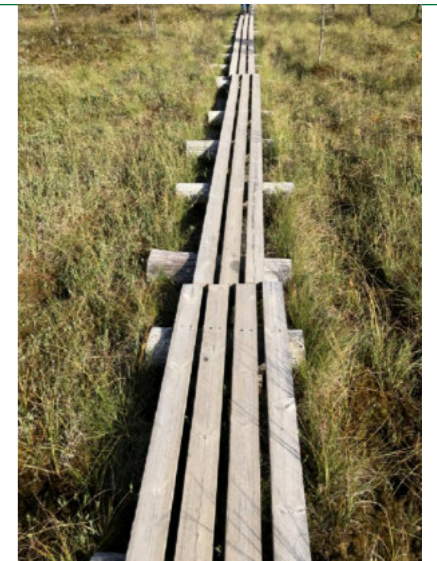
4. An upgraded trail with the existing trail left in situ and still providing support for the new trail.
