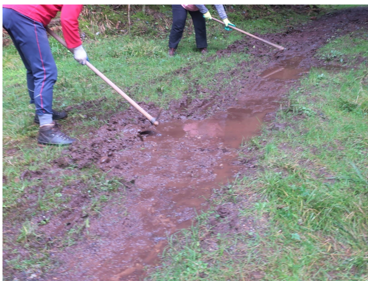
MMSE working on a very damaged track
