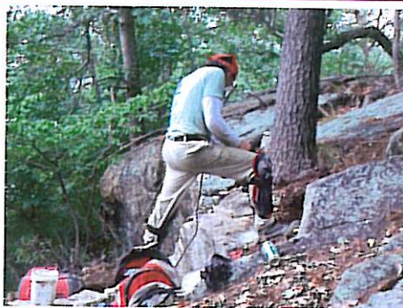
Volunteer Joe drilling rock before splitting with wedges and feathers. Joe gives two days a month to the trail, travelling up to 100 miles from his home for the weekend.
