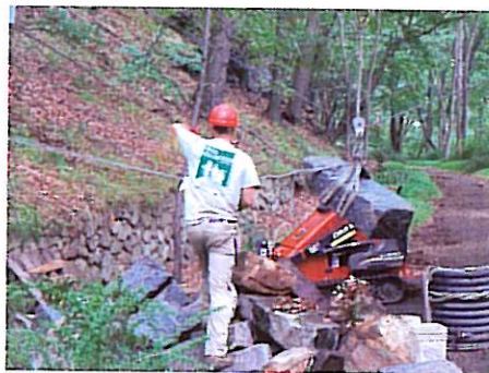
Project Manager and trail designer Ed Walsh uses an overhead cable system to move cut rock up the mountain into position as steps.
