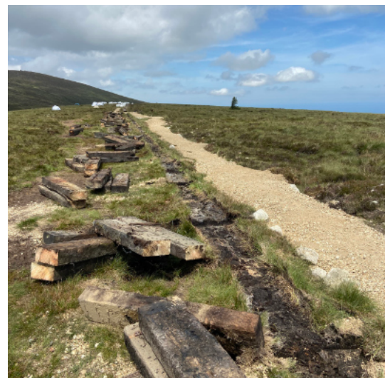
The completed section of the White Hill route. The picture also shows the removed old bog bridge.
