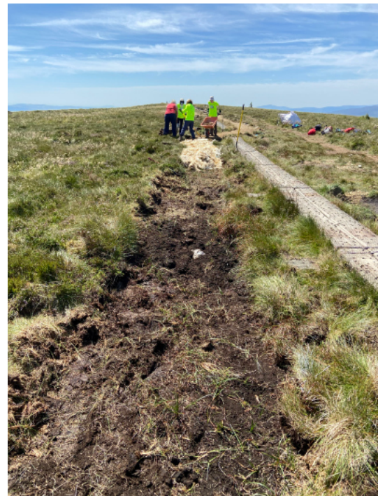
Not always "summer lark in the clear air". The weather on this exposed section of White Hill varied from scorching sun to driving cold rain, none the less but the work got done.
